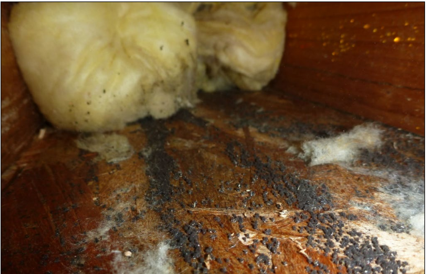
Photo 12 – Prolific fungal growth at “condensation plane” at inner face of the OSB sheathing.
