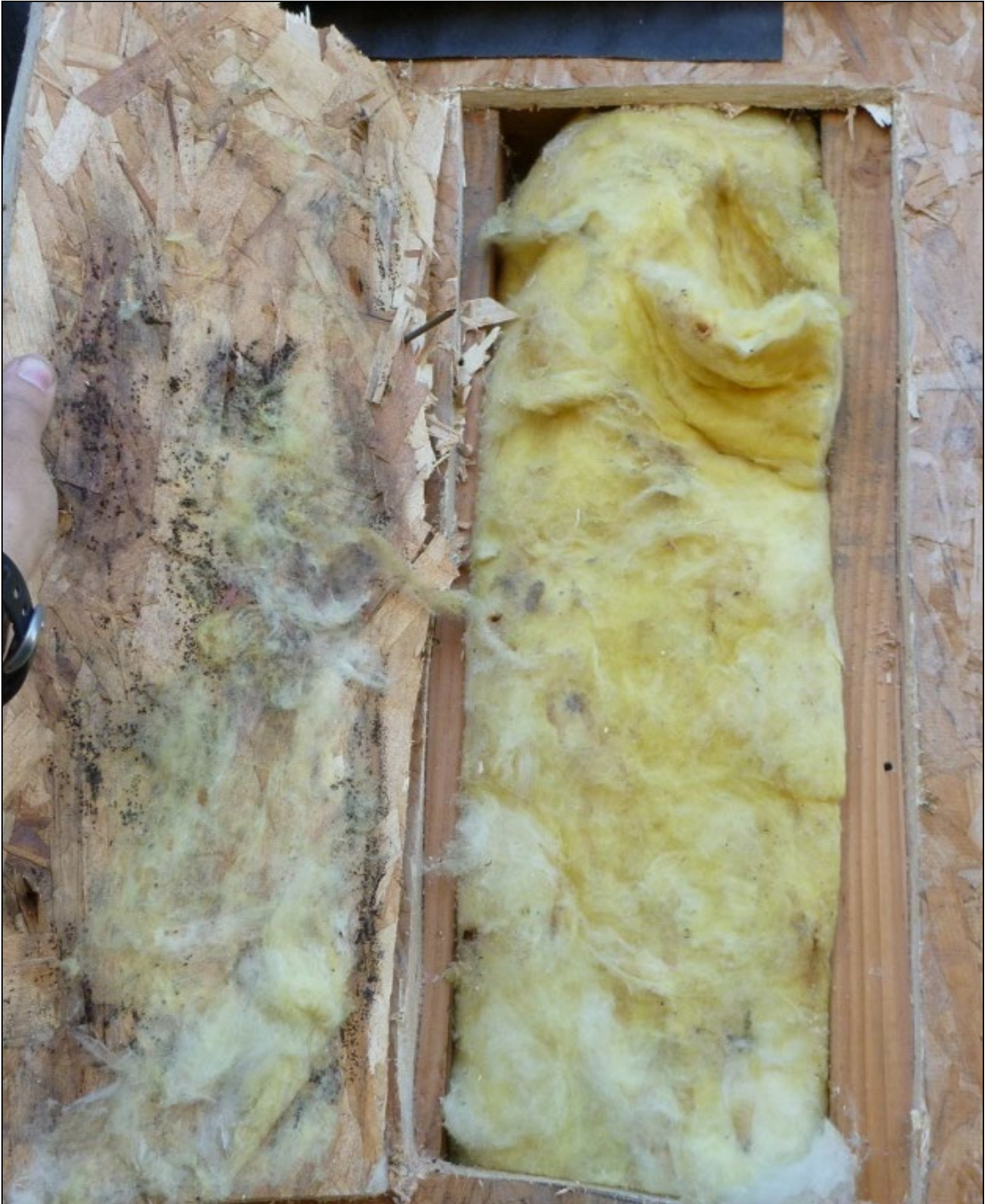
Photo 9 (same test location as Photo 10) – Fungal growth and sticky insulation remnants at inner face of the OSB panel. Again, the clean and bright exterior face of this sheathing shows no evidence of rainwater leakage.
