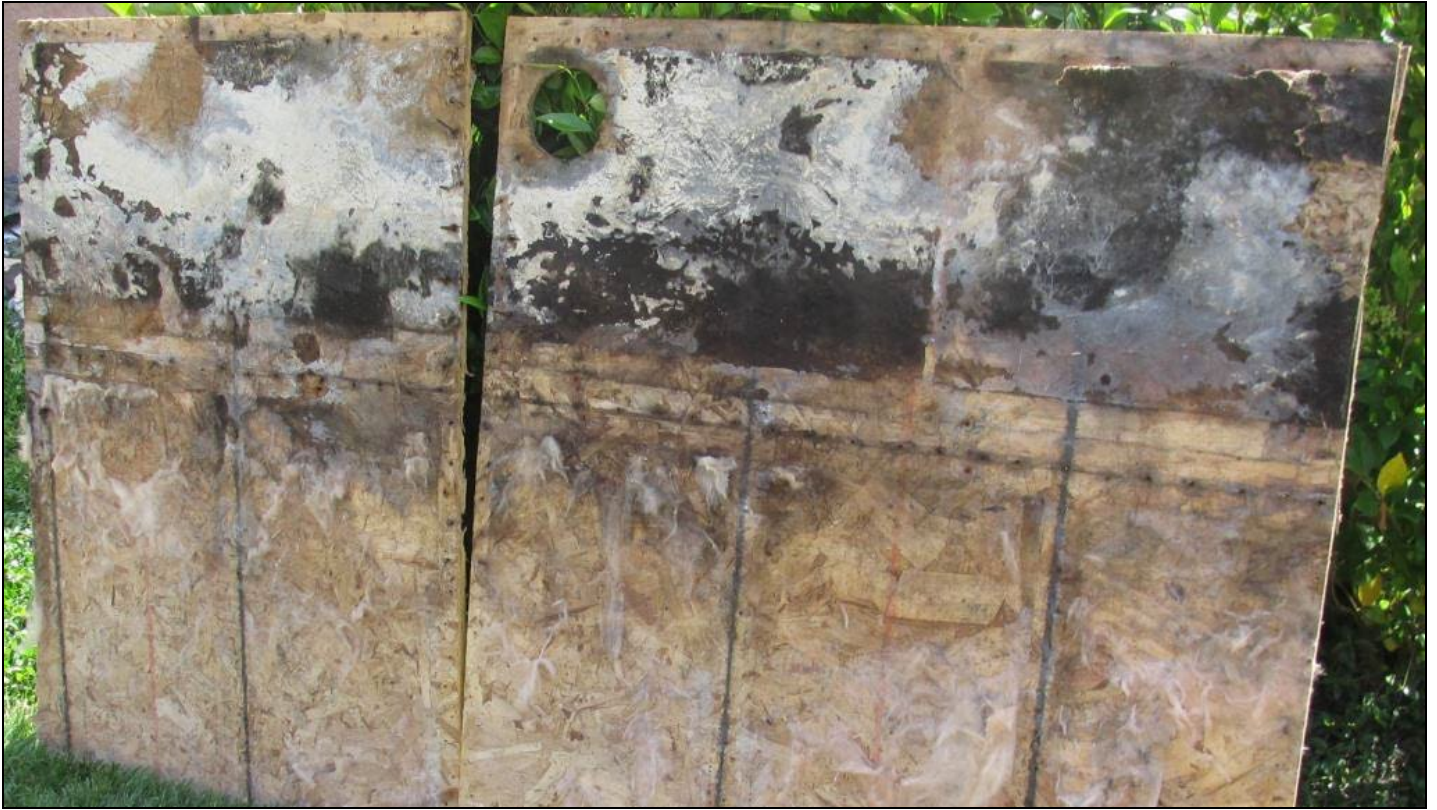
Photo 20 – Extensive fungal growth was observed at the interior face of the OSB panels where they spanned the poorly enclosed interstitial joist bays.
