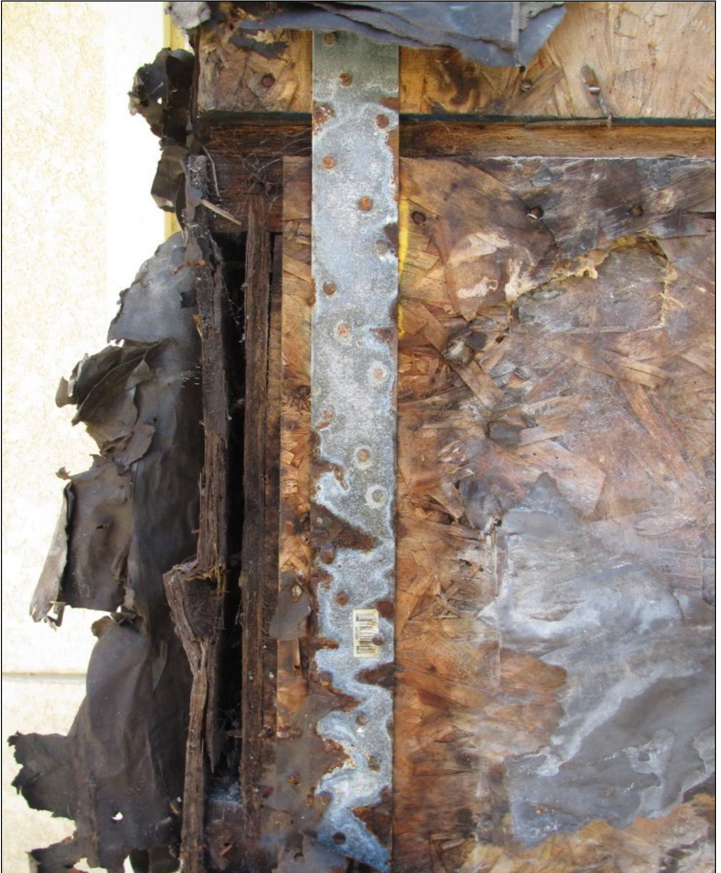
Photo 18 – In particular, the exposed deterioration and damage corresponded to poor rim joist enclosure practices.
