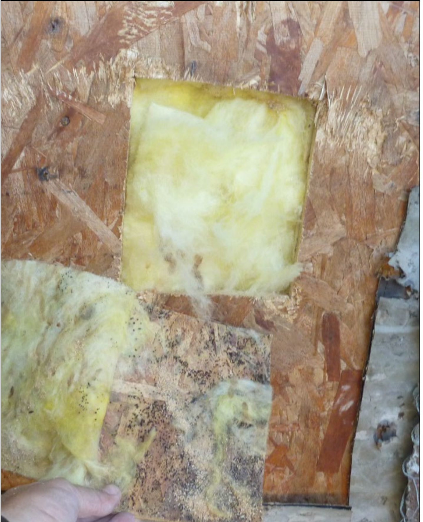
Photo 7 – The clean and bright exterior face of this OSB sheathing shows no evidence of rainwater leakage.
