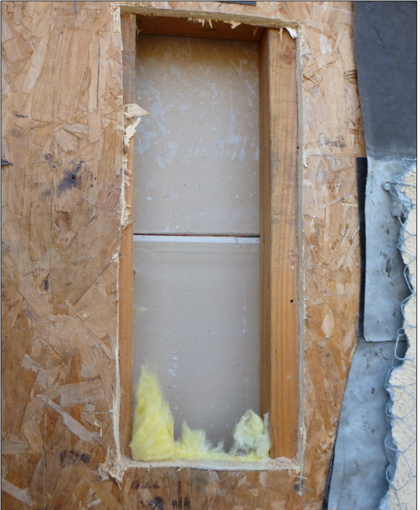
Photo 10 (same test location as Photo 9) – Because this joint was not fire-taped, contrary to code, pressurized air from the semi-conditioned interstitial space can flow (via Dr. Lstiburek’s “wind tunnel” effect) down into the cold-in-winter stud bays.
