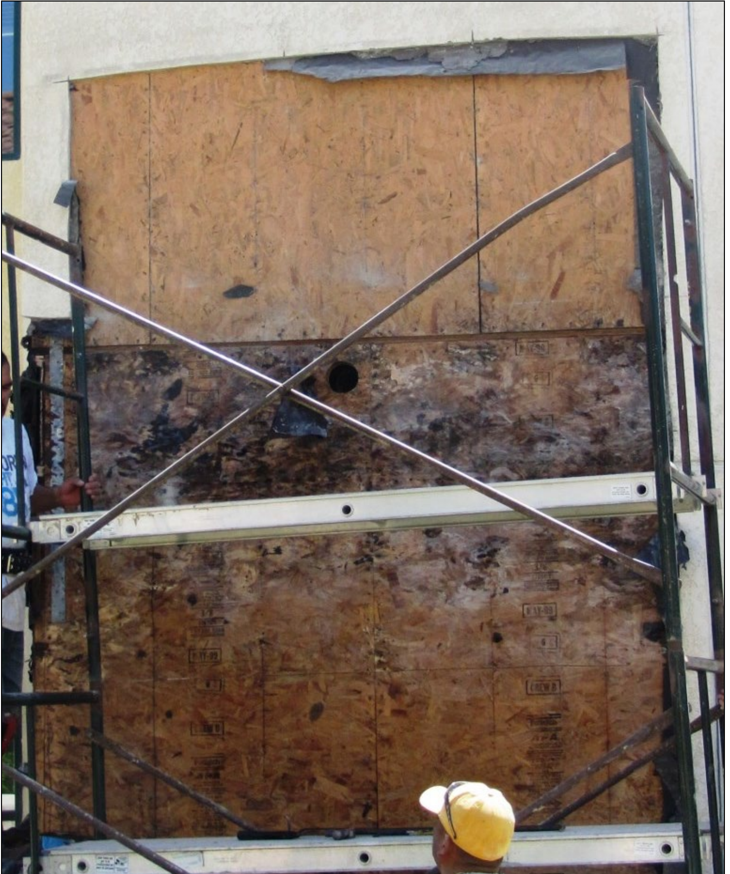
Photo 17 – Further, the deterioration and damage were most severe where these OSB shear panels spanned the 18-inch-high interstitial joist bays above the first-floor apartments.
