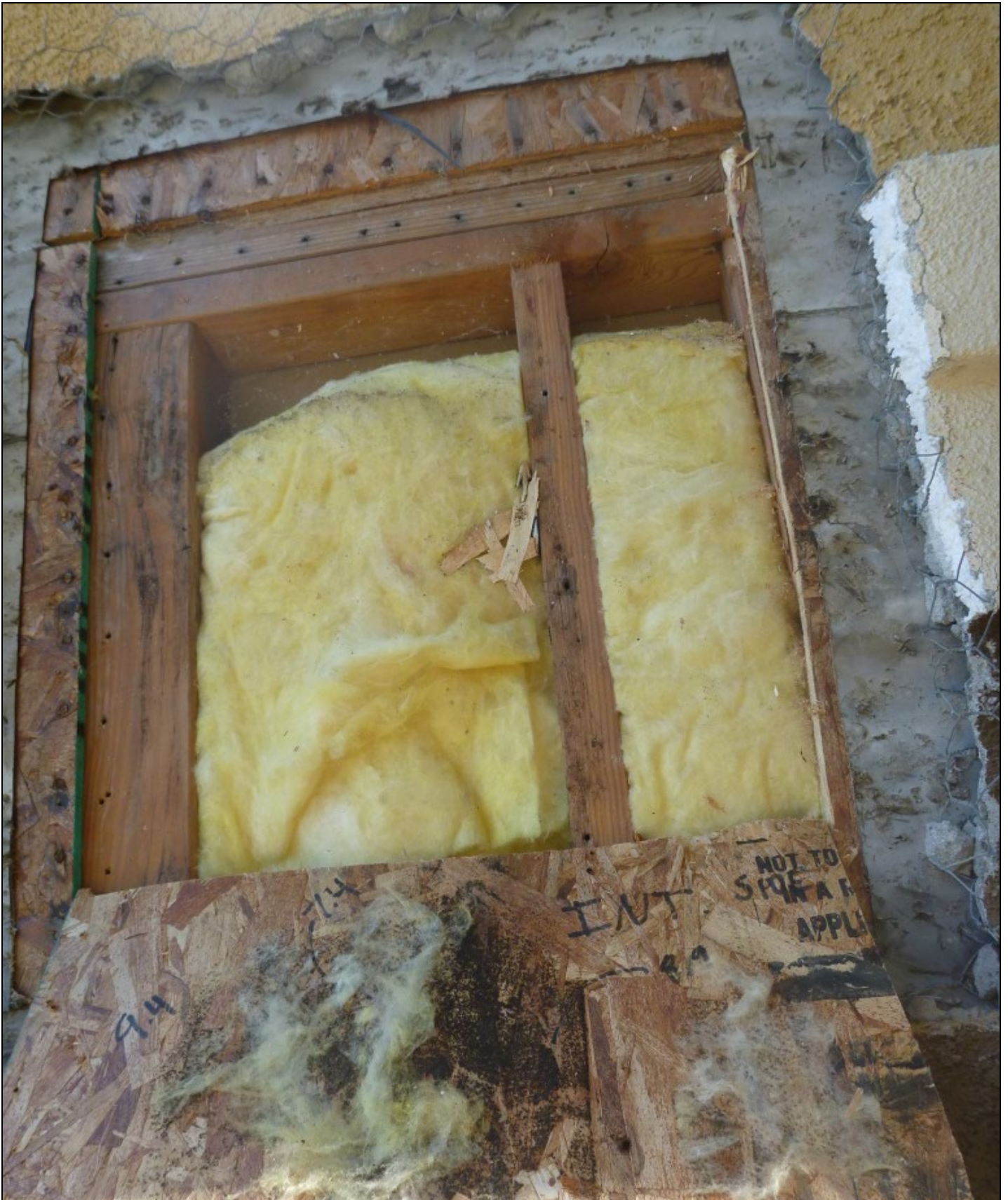
Photo 8 – Even though this OSB was dry (9.4% and 7.4% moisture content) during our summer testing, the close correlation between the fungal growth and sticky insulation is indicative of cold-weather condensation.
