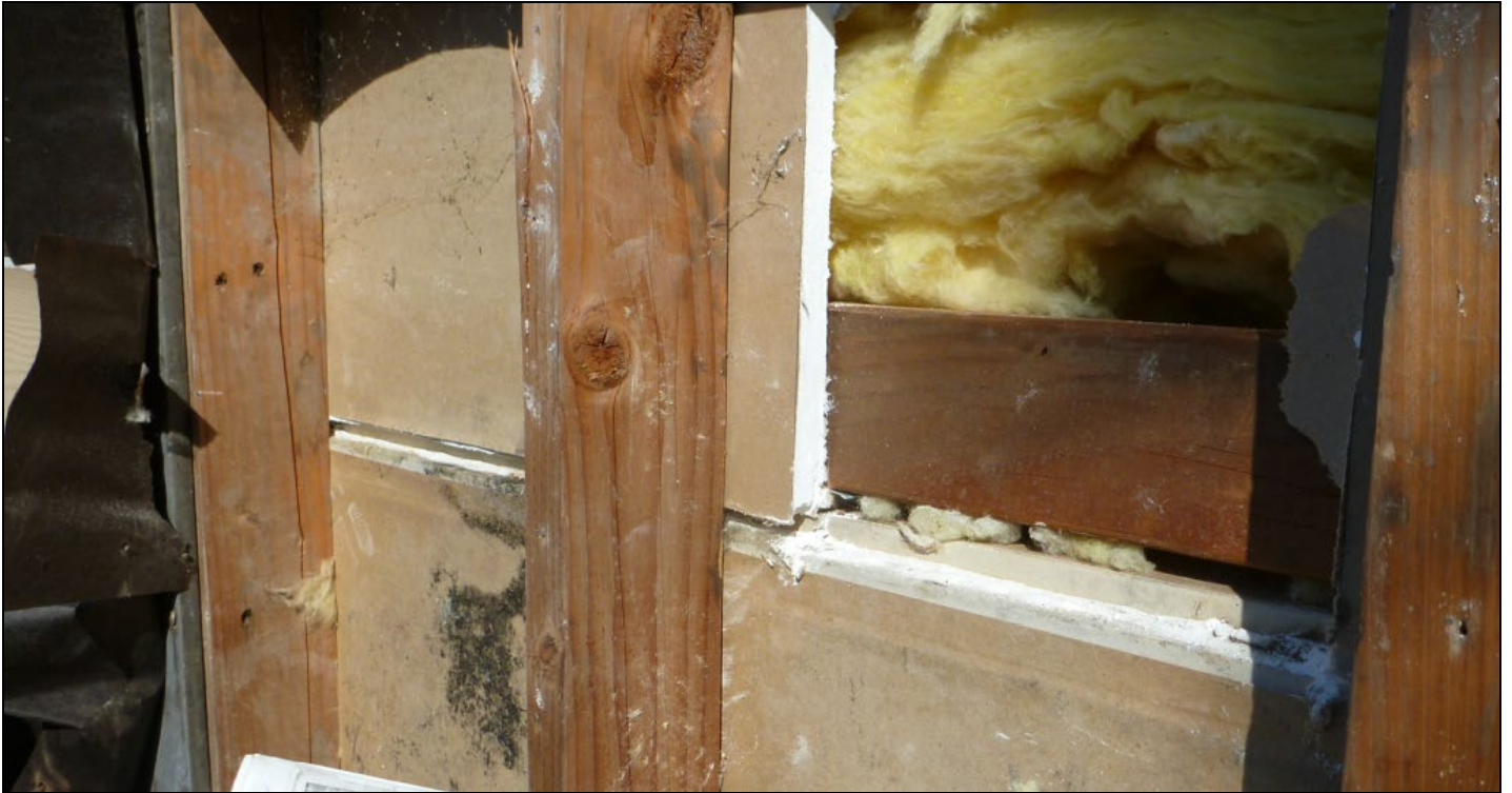
Photo 11 – The failure to fire-tape these joints between the interstitial spaces and the units below negated the code-mandated air pressure boundary. The resulting “wind-tunnel” effect produced condensation and fungal growth at the OSB panels.
