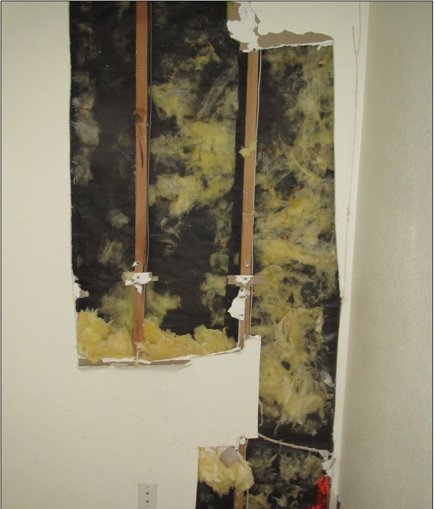
Photo 3 – These pervasive conditions (rusty line wire and remnants of the batt insulation stuck to the inside face of the building paper) indicated that the paper had been uniformly wet at times in a manner consistent with vapor condensation.
