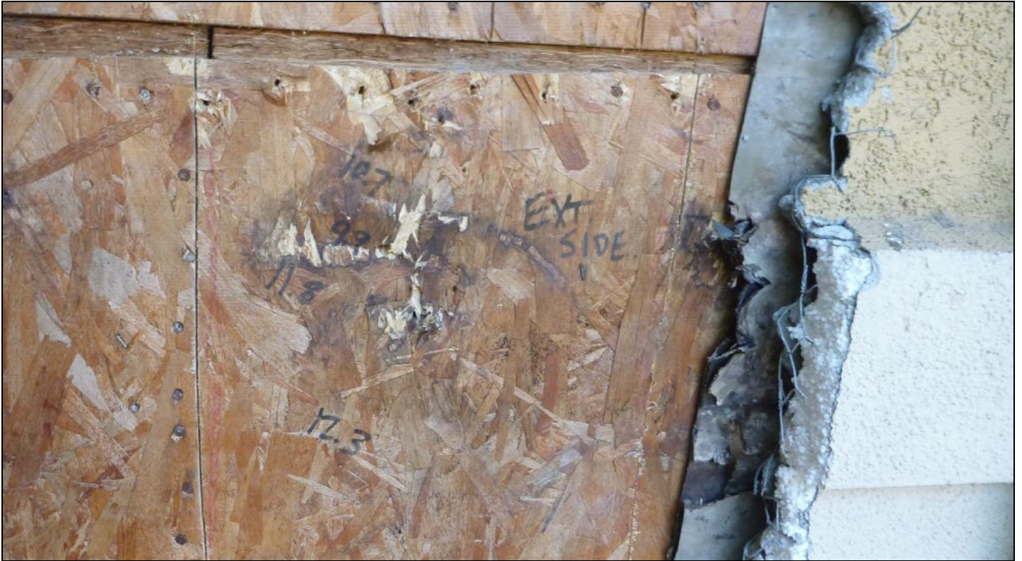
Photo 13 – While some evidence of moisture damage was found at the exterior face of this OSB sheathing, which spans the rim, far greater degradation was found at the interior face (compare with Photo 14).
