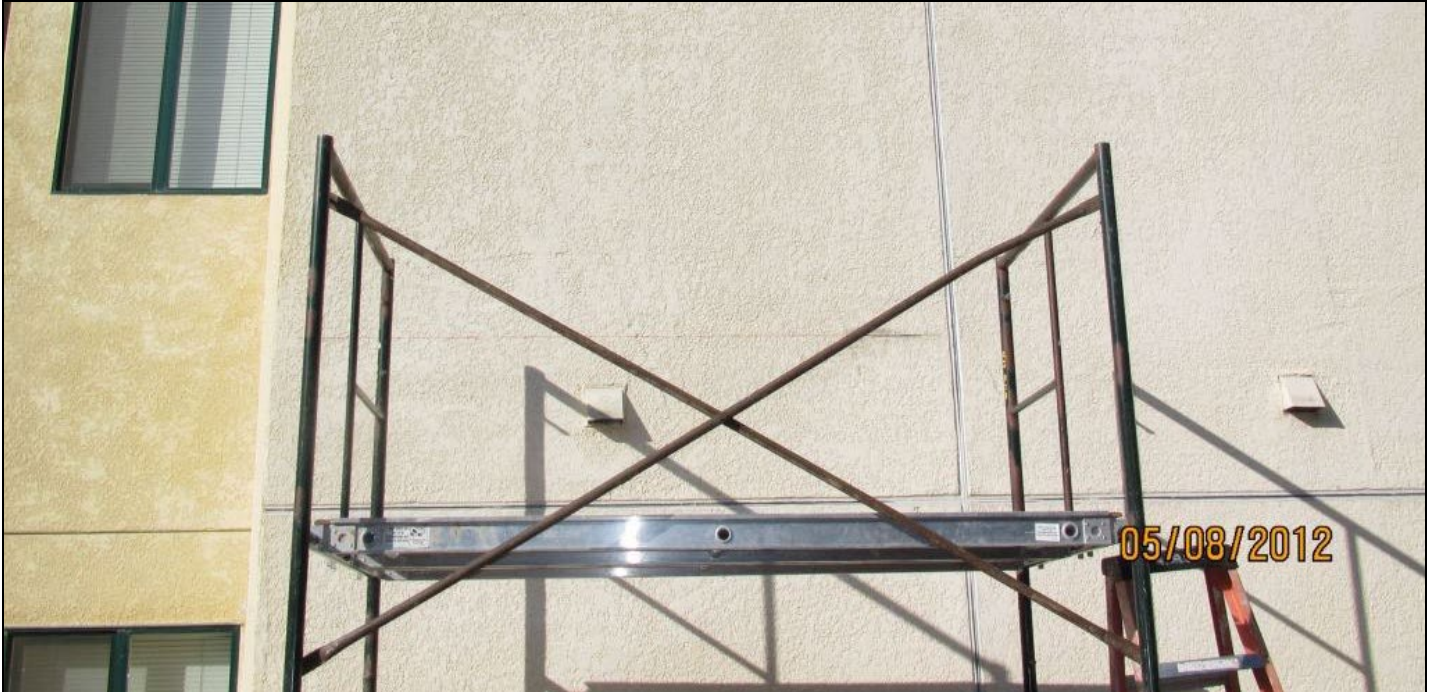
Photo 15 – Our team’s inspection in 2012 of this stucco-clad wall revealed no evidence of rainwater infiltration or decay.
