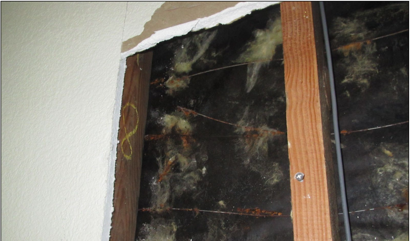
Photo 2 – The steel line wire that backed the stucco was extensively rusted and remnants of the fiberglass insulation remained stuck to the inside face of building paper. These conditions are consistent with condensation of warm humid interior air.
