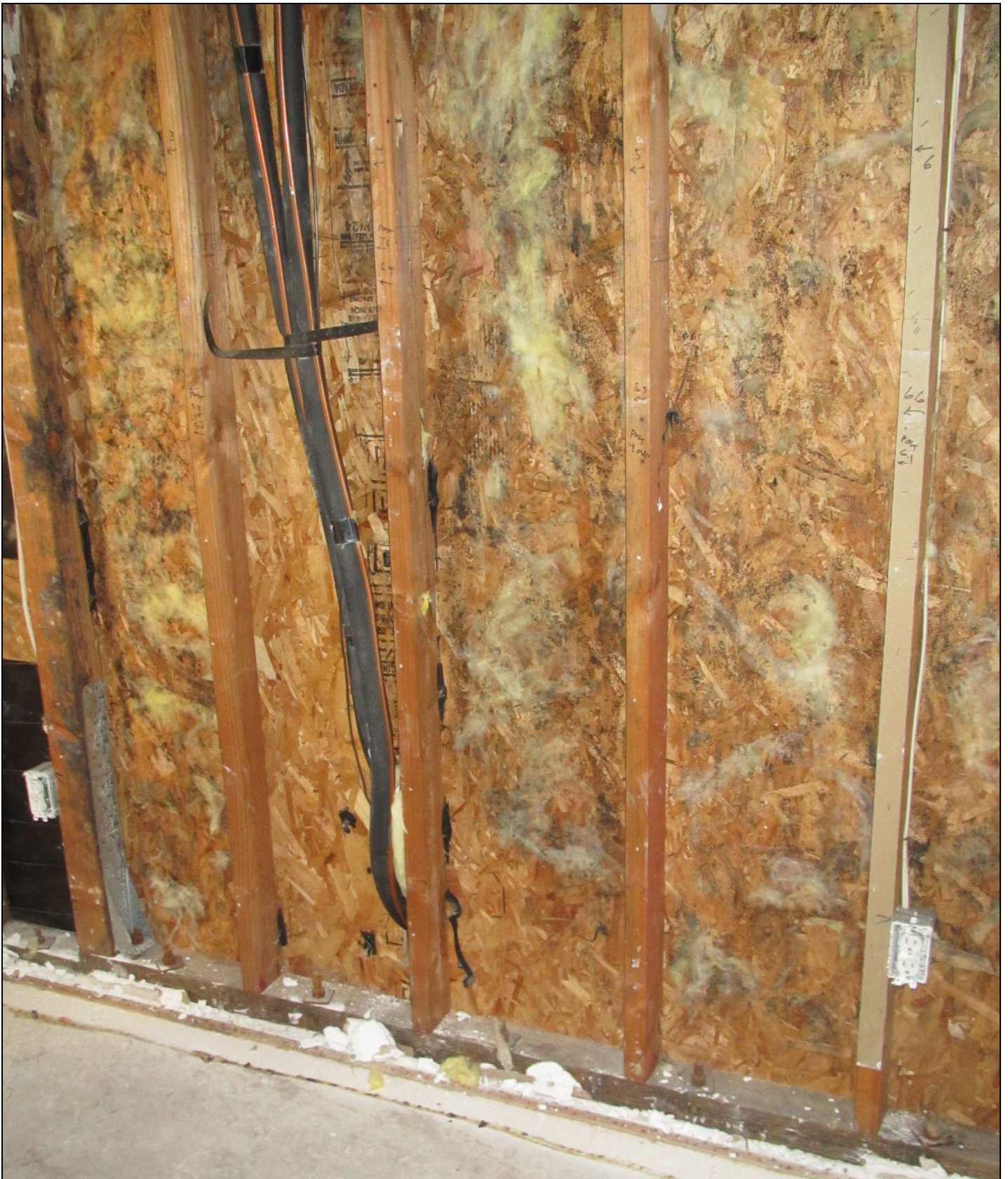
Photo 4 – At this wall, the remnants of batt insulation stuck to the inside face of the OSB sheathing indicate it has been uniformly wet at times – except at the one stud bay warmed by AC heating lines (serving both the lower and upper units).
