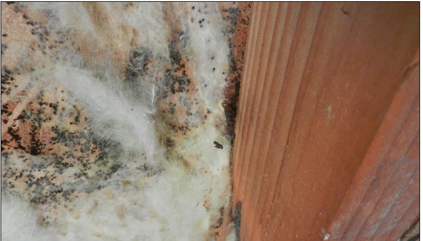
Photo 6 – Fungal growth and insulation remnants at condensation plane within stud bay at yet another exterior wall.
