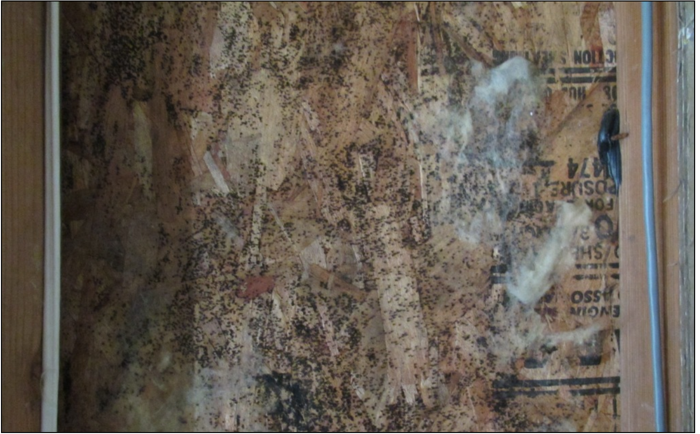
Photo 5 – Prolific fungal growth and fiberglass insulation remnants within stud bay at a different exterior wall.
