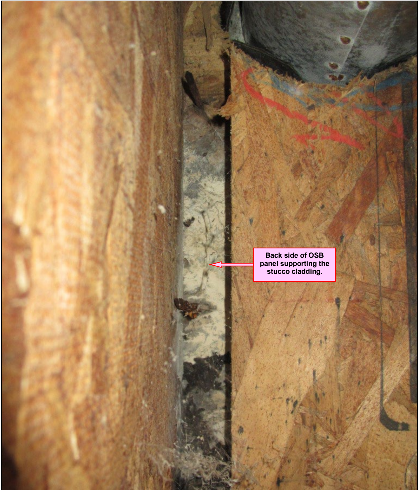
Photo 19 – At all buildings, the most severe damage was found at the poorly enclosed rim joists at the interstitial space above the first-floor apartments.
