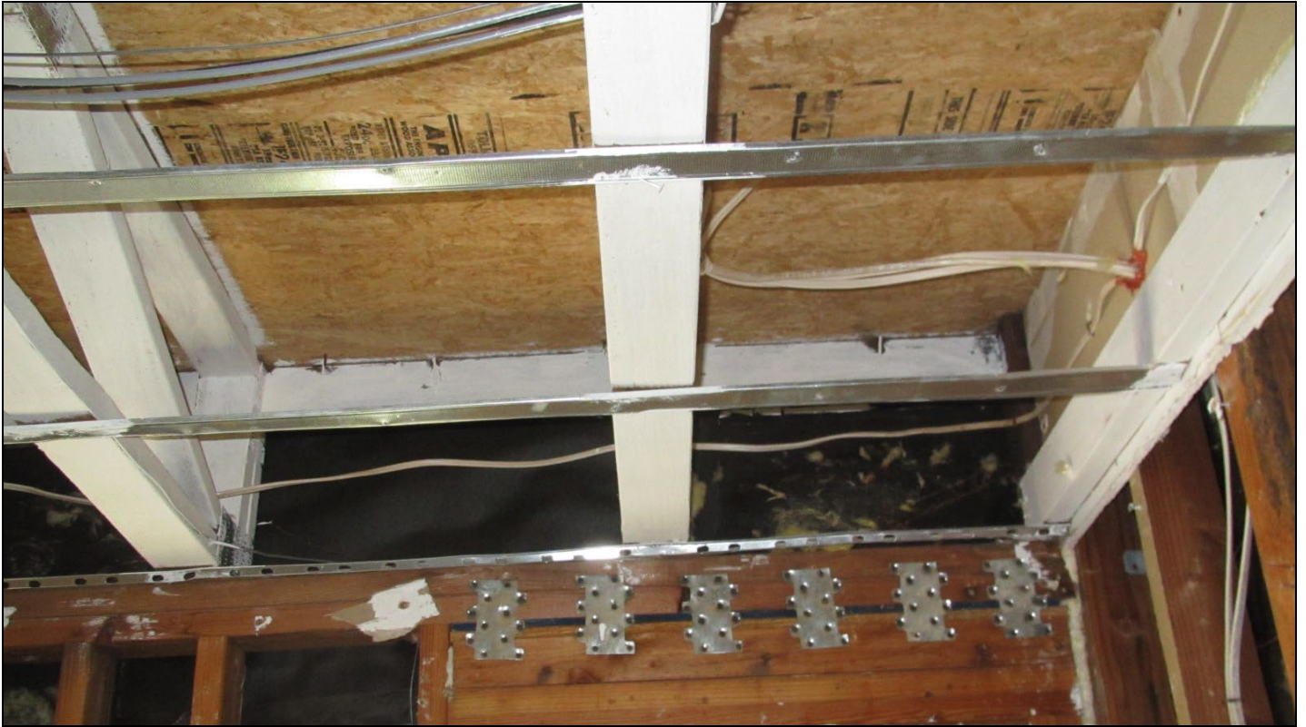
Photo 1 – No rim/band joist or exterior sheathing provided at the “open web” floor joists. Instead, upon insulation removal, we found the inside face of the asphaltic building paper serving the stucco cladding (installed over steel line wire per Photo 2).
