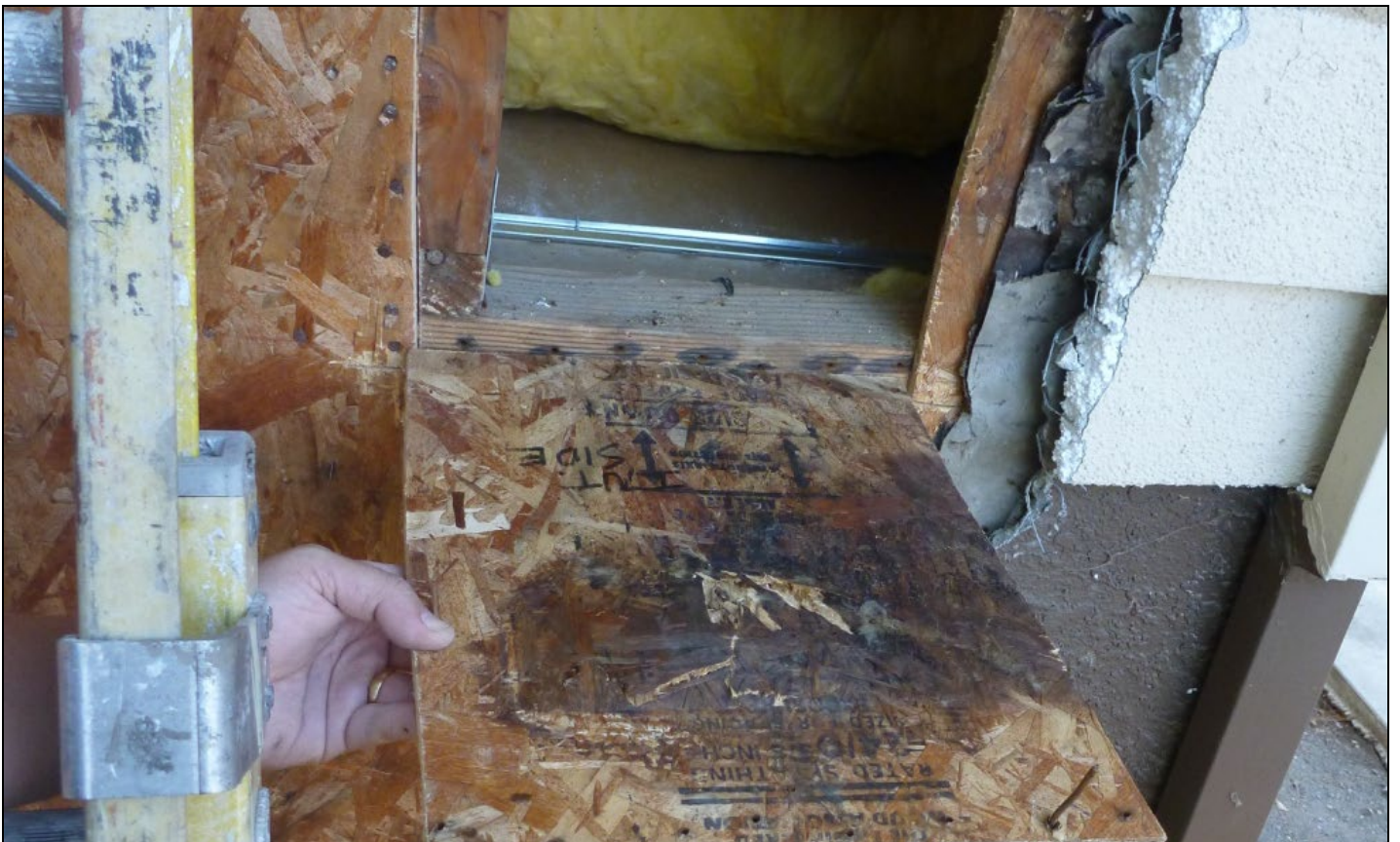
Photo 14 – In conjunction with Photo 13, this photograph conclusively demonstrates the deleterious effects of vapor condensation at the interface between the semi-conditioned interstitial air and the cold-in-winter rim.
