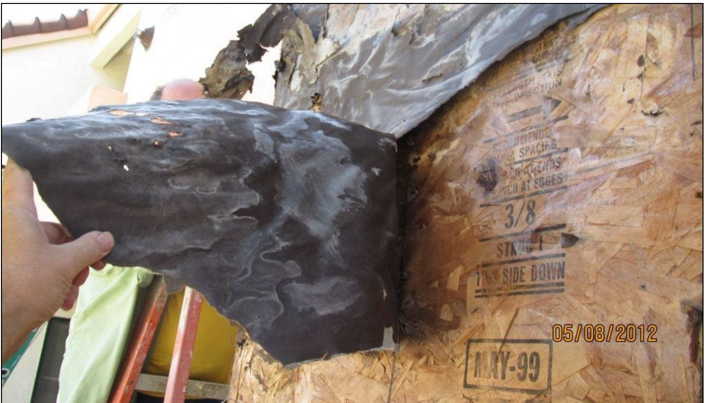
Photo 16 – However, despite the dry sunny weather, free moisture still was found behind the asphaltic building paper.
